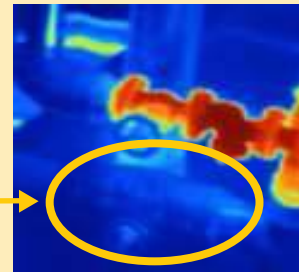
Heat losses (heat camera detection) Isolated valve shows zero heat emission
