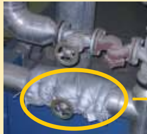
Non-isolated valve above Isolated valve in circle
